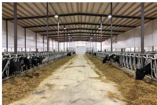
Figure 77. Cross ventilation system with curtain baffles to direct fast-moving air into the resting area
