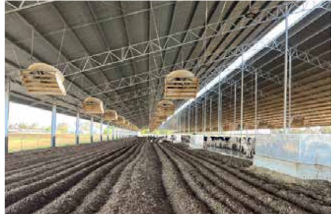
Figure 41. Mechanical ventilation (fans) – fans hung high enough to avoid equipment operating in bedding area
