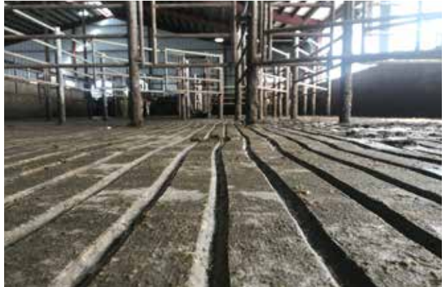
Figure 70. V-shaped groove patterns should be avoided as they result in more slips and an increase in lameness
