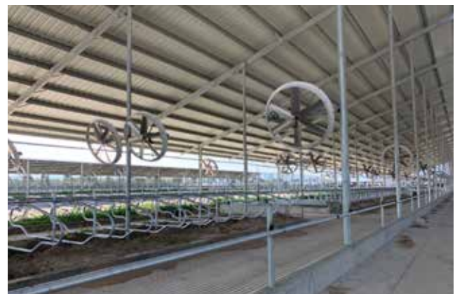
Figure 76. Fans over freestalls and the feeding table
